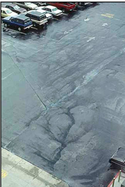
Parking lot oil entering storm drain.
