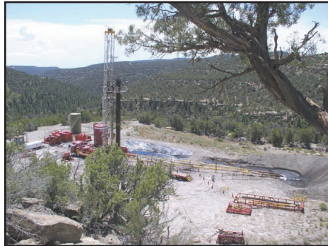
Figure 17 · The flare pit (left) and overflow pit (right) collect drilling fluid.
