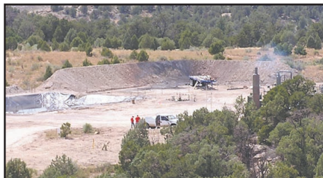
Figure 18 · A berm constructed around the flare pit blocks flares that may occur during drilling.
