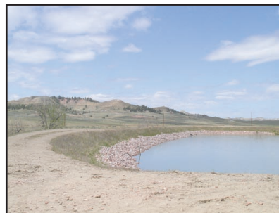
Figure 25 · Riprap used to protect the windward side and dam face of a CBM storage pond from erosion caused by wave action.
